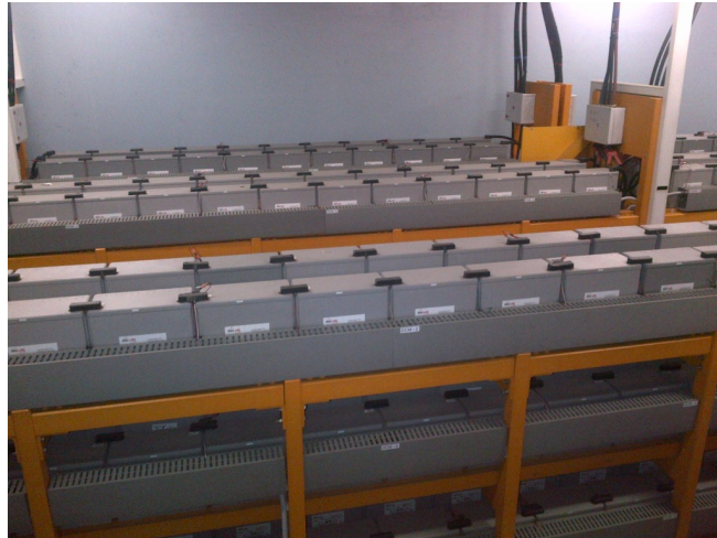
Cellwatch Battery Monitoring installed at SNCF
